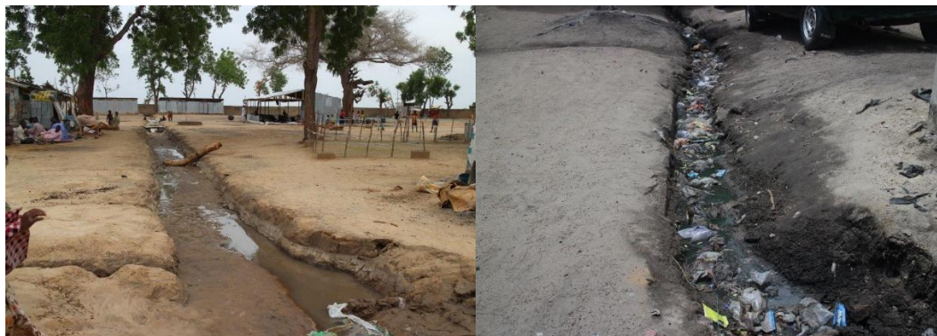
Figure 45: New irrigation channel in camp (left) and clogged channel in urban host community (right)
