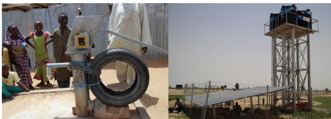
Figure 16: Handpump (left) and elevated storage with solar powered borewell (right)
