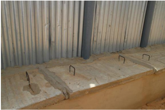
Figure 28: Sealed service slab with vent pipe not properly separated from the service slab
