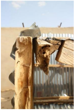
Figure 39: Termite damage to latrine superstructure
